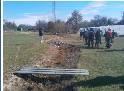
Real Food Farm – Clifton Park site storm-water management projects – underground cisterns and 4,000 sf bioswale
