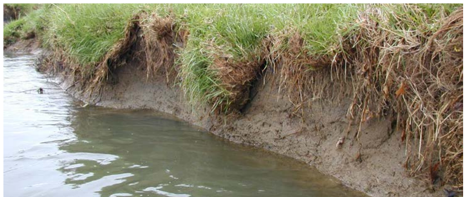
Figure 1. Single-arm vanes redirect flows from banks, reducing erosion caused by high flows.
