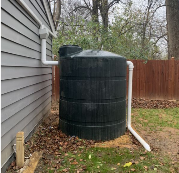
Figure 3. A cistern installed through the RainScapes Rebate Program.
