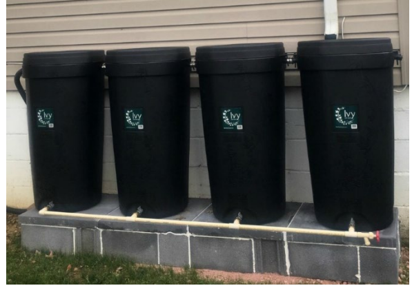
Figure 3. Four 50-gallon rain barrels connected together and installed at a residential property.
