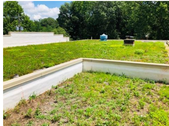
Figure 16. A green roof at the Town of Forest Heights' municipal building. This is an example of a green roof. This project was not funded through this program.
