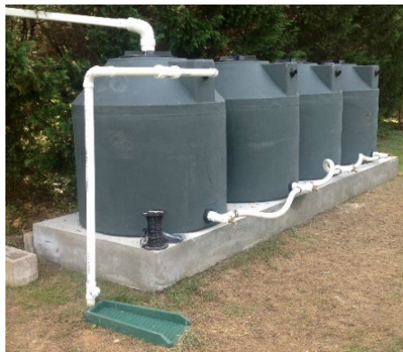
Figure 4. Four 305-gallon cisterns connected together and installed at a residential property.
