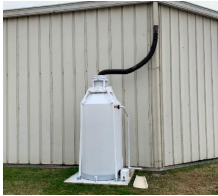
Figure 5. A 250-gallon cistern installed at a nonprofit organization.
