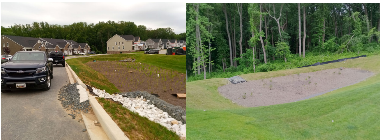
Figure 3. Photos of ESD stormwater BMPs that were installed in the UTLP watershed during the monitoring project.
