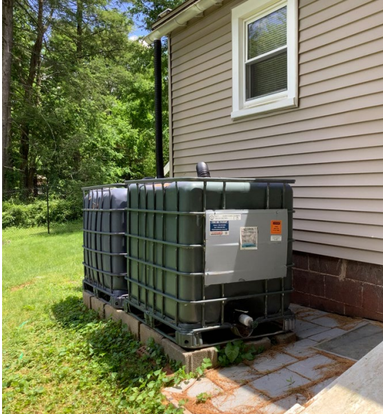
Figure 3. Cisterns installed through the City of Gaithersburg RainScapes Reward Program.
