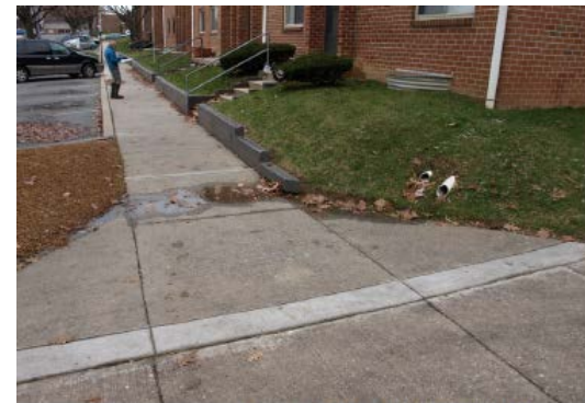
Drainage Conflicting with Walkways
