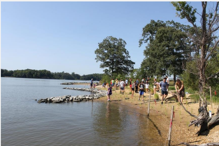
This living shoreline project restored a significantly-eroded section of the Camp Letts campus.
